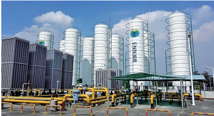
Company Natural Gas Plant Station
