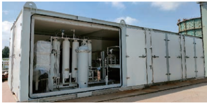
Natural Gas Skid-mounted Hydrogen Production Project
