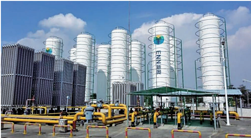
Company Natural Gas Plant Station
