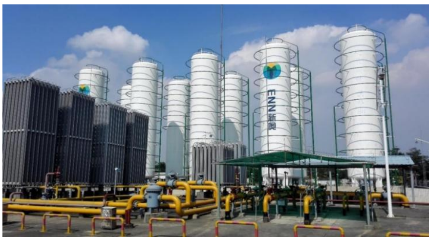
Company Natural Gas Plant Station
